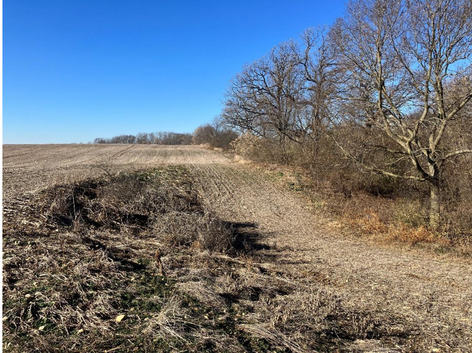
Photograph 17: Photo point - eroded slope at north of farm field
